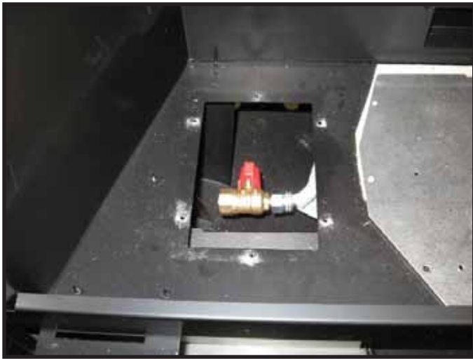
Figure 11.3 Gas Fitting Access
