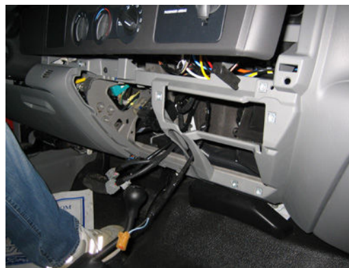
Current view of installation
