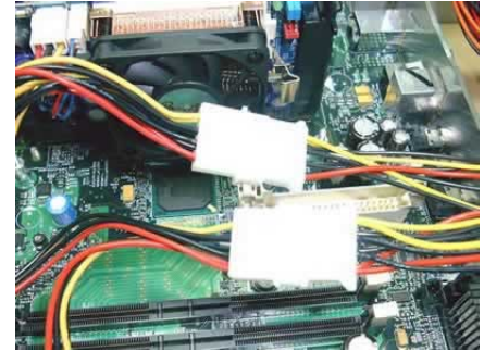
The connected cables for two PL-P3/SMPs.
