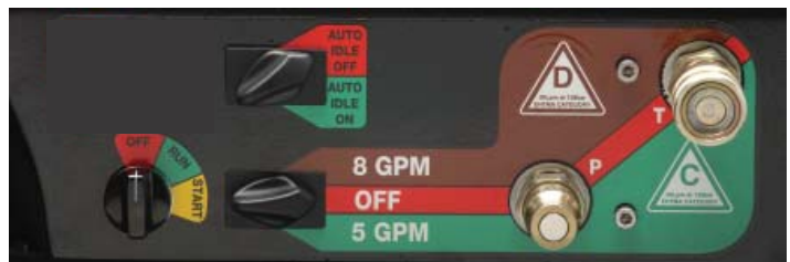
Figure 1. Panel Control Valve
