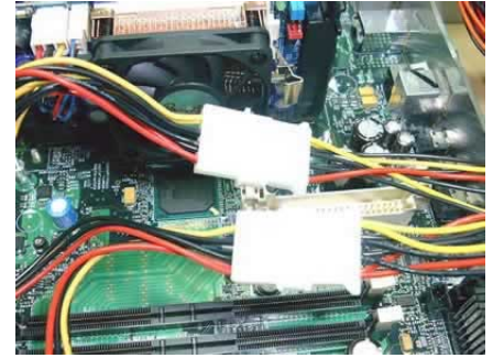
The connected cables for two PL-P3/SMPs.
