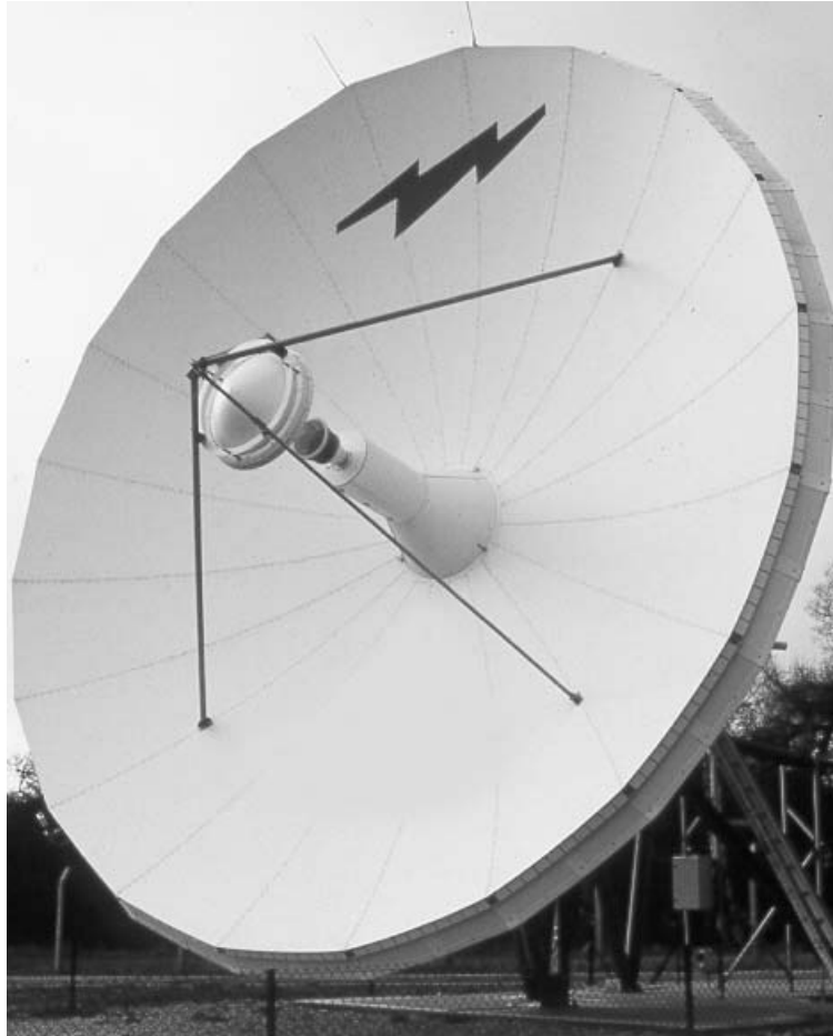
9.3-Meter Earth Station Antenna
