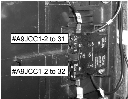
Figure 28: Right side of Motor Contactor
